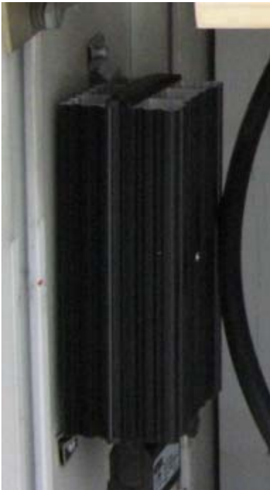
Heater Mounted in Cabinet
